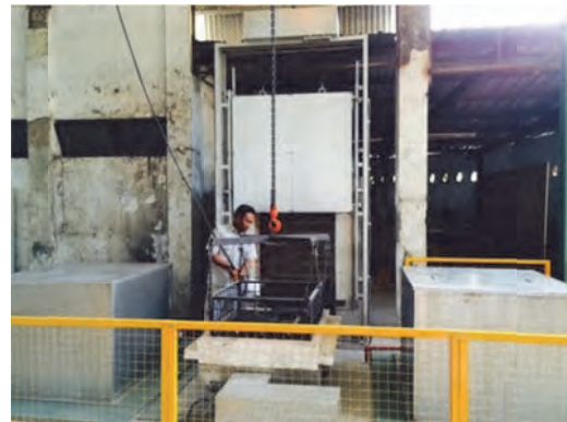
⑥ Heat Treatment Furnace installed in the MIDC
