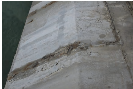
Corrosion. The fairing is not a structural member but it is better to remove the rust and repaint immediately.
