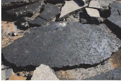
3. Removed pavement of North Lane, west side span. Back side of pavement. This black color indicates healthy adhesion to steel deck.
