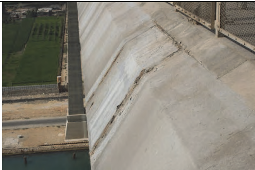
Site welded fairing part is severely corroded.
