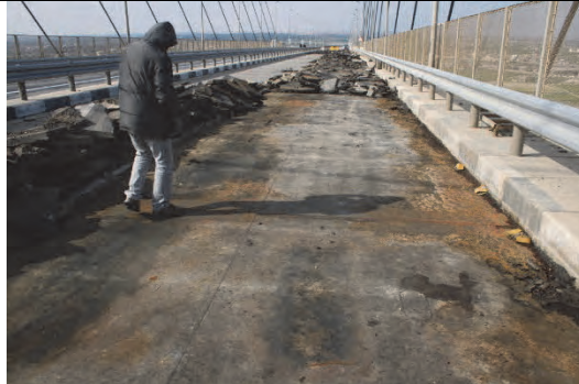
The corroded areas are on both sides which are below the cracked pavement areas. The center area is healthier.
