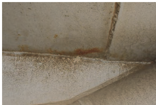
3. Some rust near pipe fixing structure.
