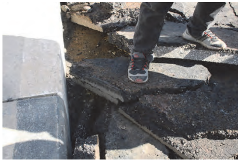
5. North side curb and some rust of steel deck plate is seen.
