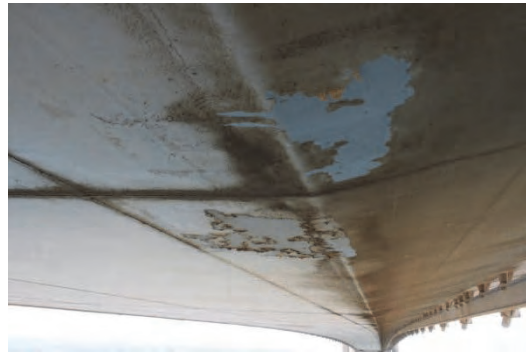
2. The same kind of rust as Photo 24. The all surfaces are covered by very fine sand, which may include salt particles.
