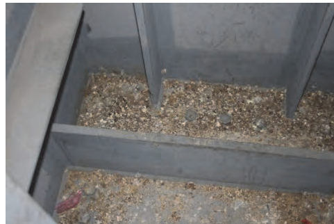
6. Entrance of Box Girder. Bird droppings. This should be removed.
