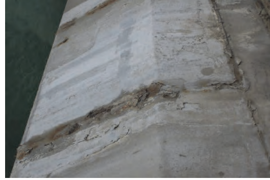
8. Corrosion. The fairing is not a structural member but it is better to remove the rust and repaint immediately.
