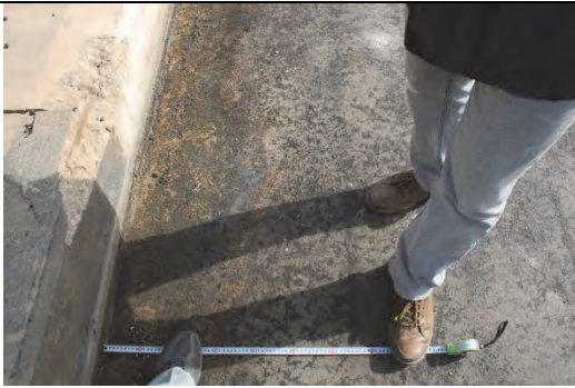
The welding line of R4 U-rib below the steel deck, which is 64cm apart from the curb is visible on the left of the brown shoes.
