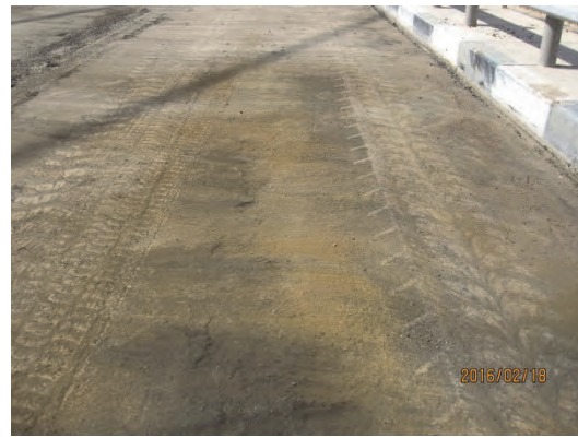
2. Corrosion of the surface East side (North lane)
