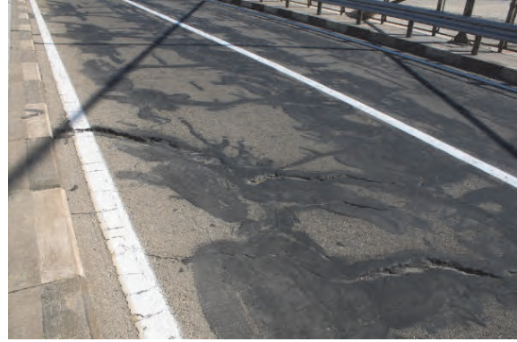
2. This is the same photo as Photo 1 from 28th Day Report. The same large cracks as Photo 1.
