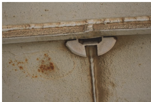
4. Some rust near site welding. Bottom plate is also site welded.
