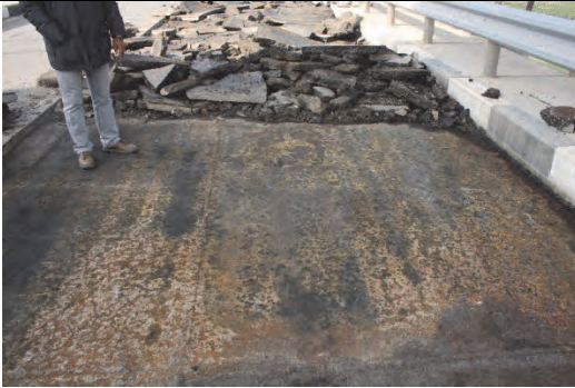
Corrosion near the west tower and on the North Lane.
