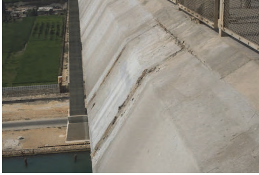
7. Site welded fairing part is severely corroded.
