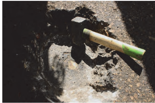
16. Size of the hole on the deck
