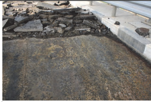
Corroded area near the west tower. This may be worst corroded.
