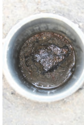
2. P11, bottom surface is broken by hand and rusty deck plate appeared.
