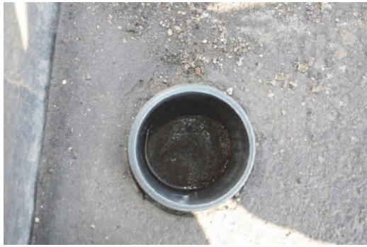
1. P11, Some water is observed and the bottom surface is swollen.
