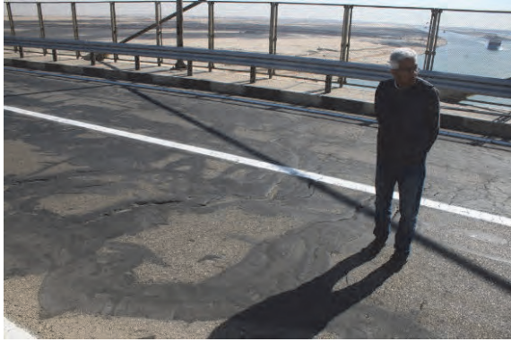
1. This is the same photo of 28th Day Report. Large cracks at center of center span on South Lane near 3rd cable from the longest west side cable. It seems the pavement is flowing. The reason is unclear. 3rd cable is fixed near D58 Diaphragm. The inside around D58 was examined.
