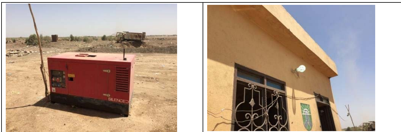
Fig. 4-10 Generator and Light Equipped by KCC
