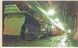
Photo 2 Continuous belt conveyor in the tunnel
