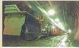
Photo 2 Continuous belt conveyor in the tunnel
