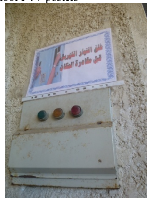
Figure 23: An Example of a Safety Poster “Switch off After Use.” (School T)
