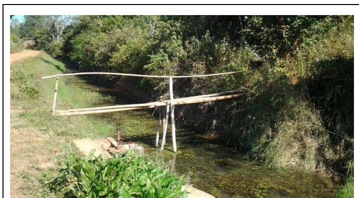
A rustic wooden bridge which was constructed by villagers by themselves. A foundation is unstable and dangerous and is not suitable for transportation of heavy agricultural produces from farm plots. (Hopon Irrigation Scheme, Shan State)
