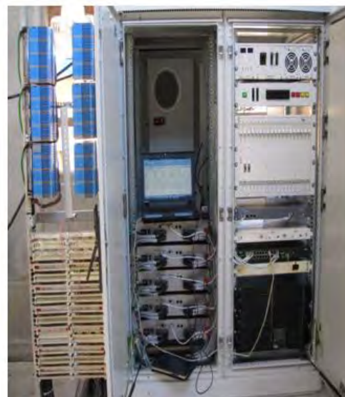
Front View of equipment inside FTTC
