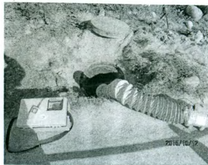
GAS DETECTOR and Exhaust Fan USED INSIDE
