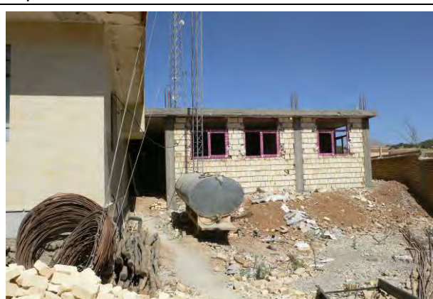
Bazoft guesthouse construction: Materials for the construction were purchased by the project; the guesthouse was constructed by NRWGO (June 2011, Telurd town in Bazoft area)
