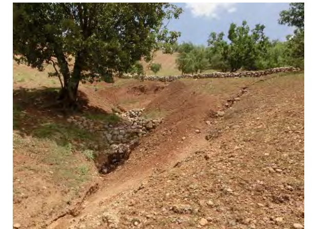
Forest and Rangeland sector: Check dam maintenance; after heavy rain, a gully newly formed from the upper side of the dam body (April 2015, Durak Sofla village in Bazoft village)
