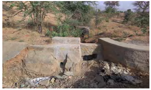
Breaching of canal
