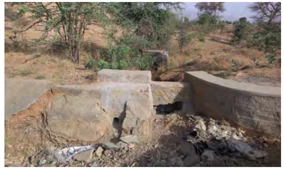
Breaching of canal
