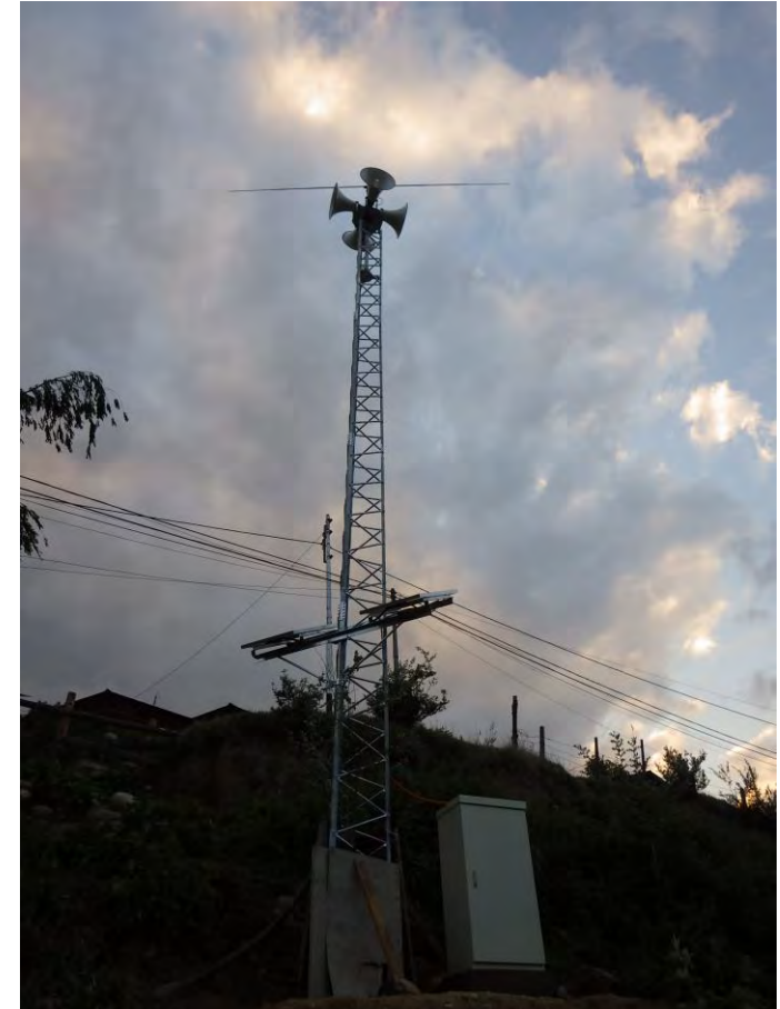
Siren Tower with Solar Panel and Outdoor Equipment Rack (Sample for reference)
