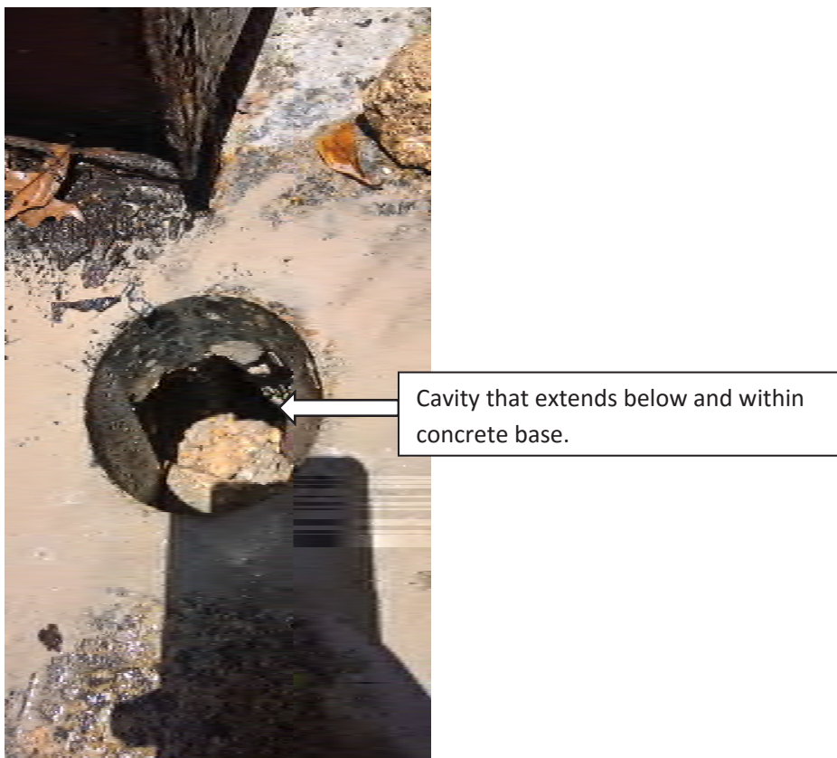
Figure 11. Picture showing entrance to cavity found at second boring site
