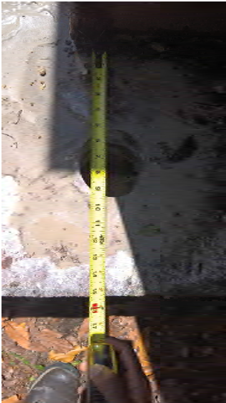
Figure 12. Picture location of third boring in southeastern corner of concrete base
