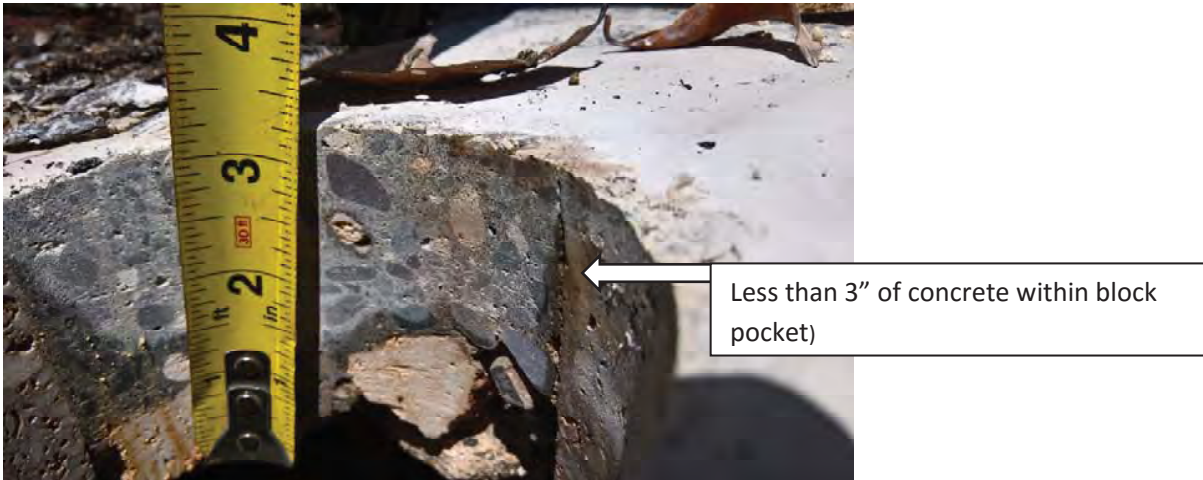
Figure 10. Picture showing thickness of partial infilling of block pocket at location of second boring
