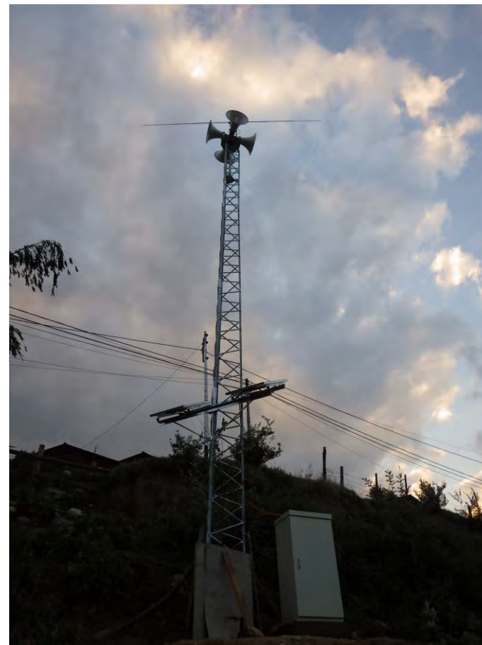
Siren Tower with Solar Panel and Outdoor Equipment Rack (Sample for reference)
