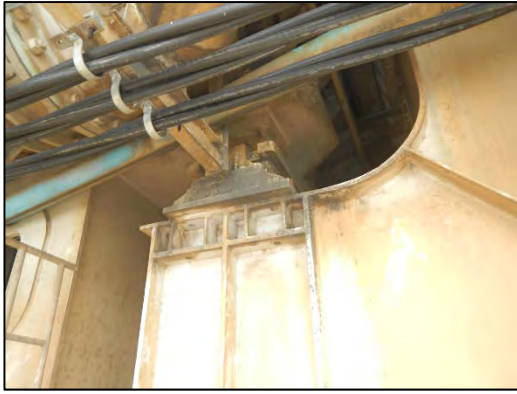
High-voltage cables attached to the steel box girder (22kv × 3)
