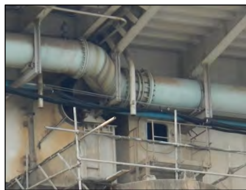
Water pipes attached to the steel box girder ( \phi 800 )
