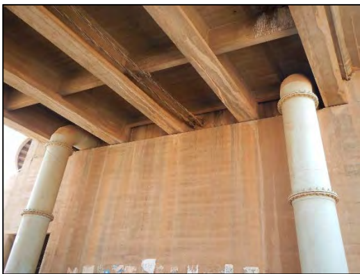
Water pipes on the wall of the pier ( \phi 800 \times 2 )
