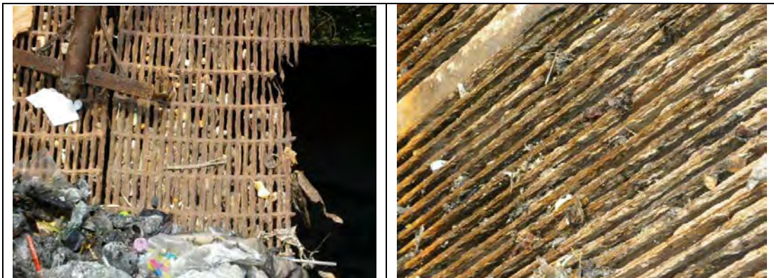
Photo R 2.2.3 Condition of Existing Bar Screen
