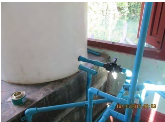
Chlorine Dosing Filter
