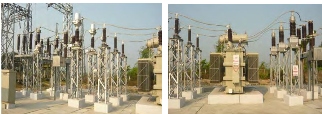
A Sample of 66/33KB Sub-station
