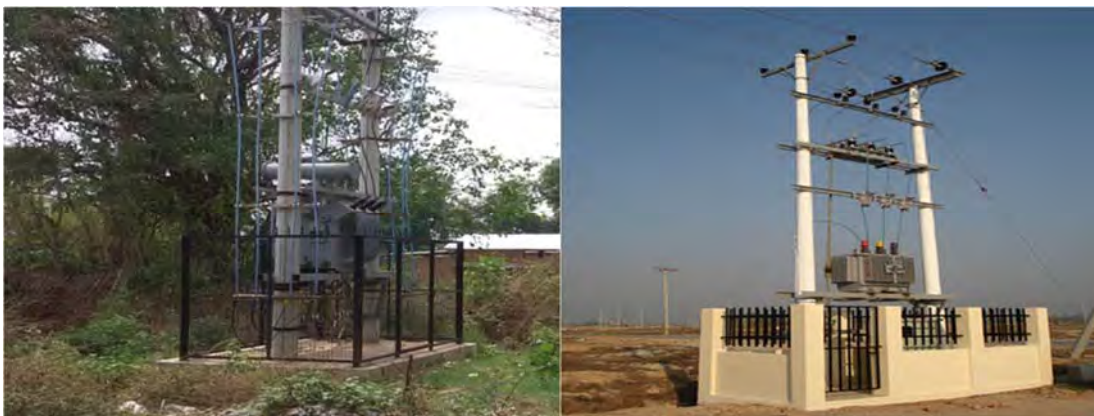
Samples of 11/0.4 KV distribution transformers
