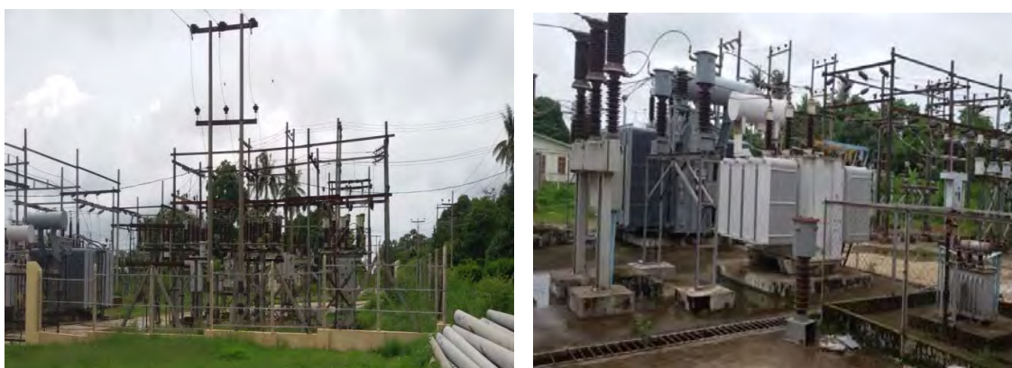
A Sample of 66/33/11 Sub-station
