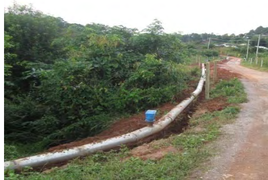
Transmission Pipe Line
