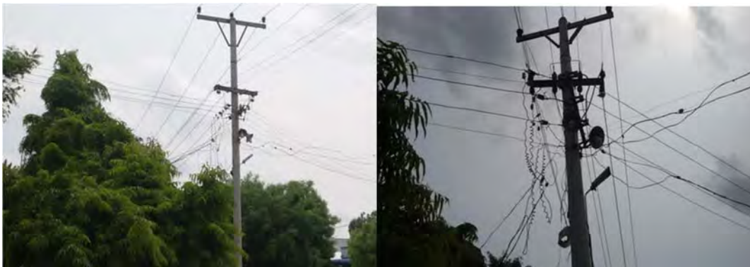
A Sample of combination of 11 KV and 0.4 KV distribution lines
