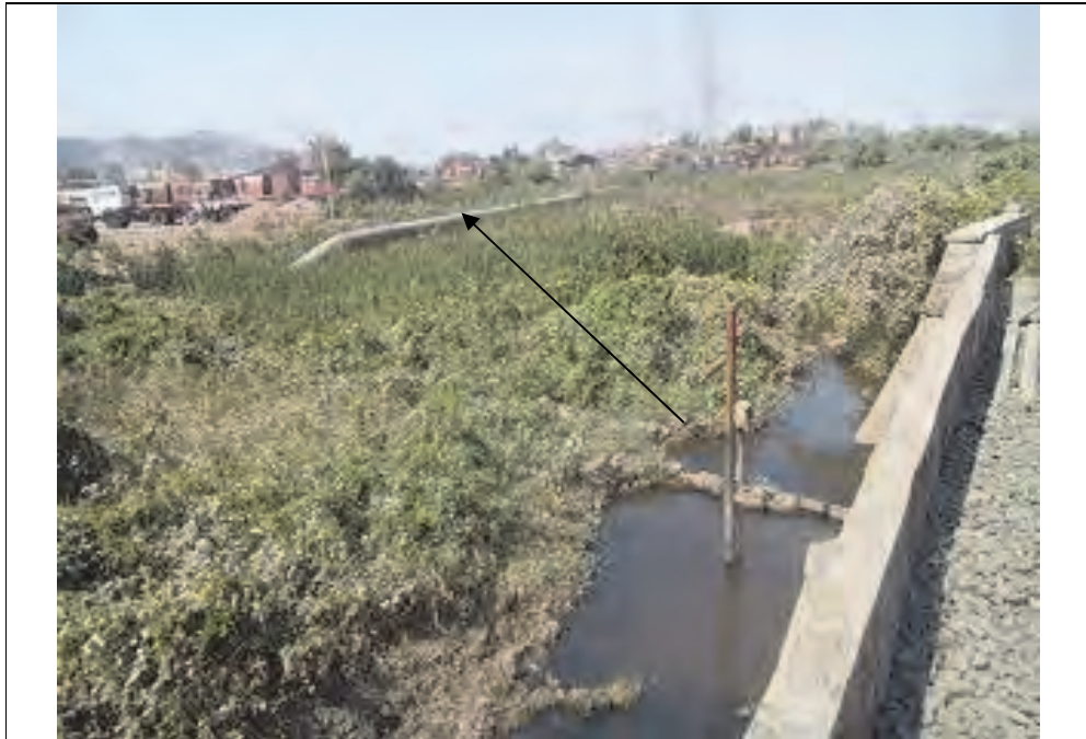
Figure 12 Water pipe line of CIDCO at Jasai Village
