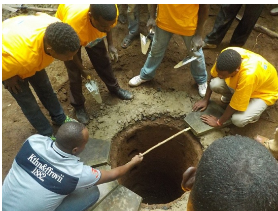
Installation of reducer blocks, taught by TVETC instructor, Mr. Tarekegn (front left) (Photo by WAS-RoPSS)
