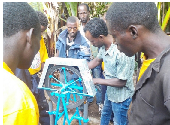
Quality check after installation by Mr. Alene, Technical Assistant of JICA WAS-RoPSS (center) (Photo by WAS-RoPSS)
