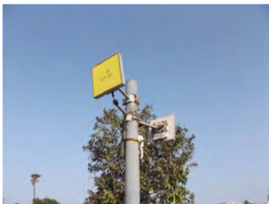
Picture 3-7 RFID Reader around CFS Entrance and Exit
