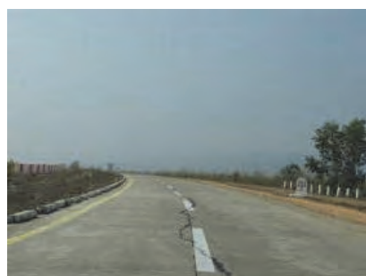
Damage of pavement
