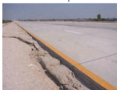
Damage of shoulder
