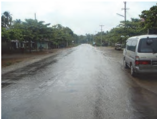
Photo-7 Road Condition on Thaton – Eindu Section
