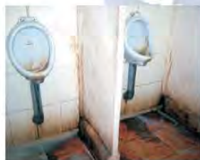
Figure 11(a): Poor condition of CTC
