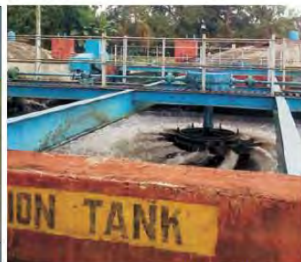
Figure 8: GCDA's sewage treatment plant at Marine Drive
