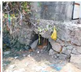
Figure 9: Inadequate septage management
