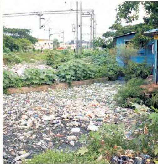
Figure 21: Garbage in open Drain
