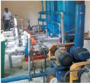
Figure 32: Hi-rise buildings-Inhouse Sewage Treatment facility
