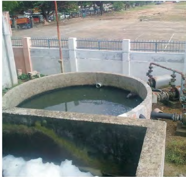
Figure 33: GCDA Sewage Treatment Plant at Marine Drive
