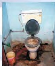
Figure 11(b): Poor condition of CTC
