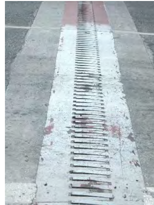
This expansion joint on the south approach bridge is maximally contracted and has collided a bit.
