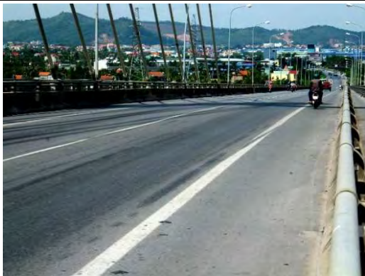
Surface unevenness has already appeared (north side).
