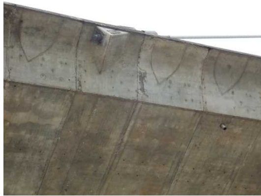
Slight concrete spalling is found on the web.
