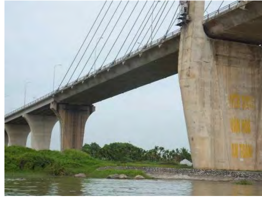
The side span box girders have been painted. The reason is unknown.
