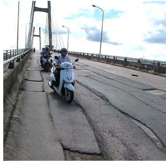
Pavement conditions of Kien Bridge in September 2014. Source: http://www.baohaiphong.com.vn/ <03/09/2014>
