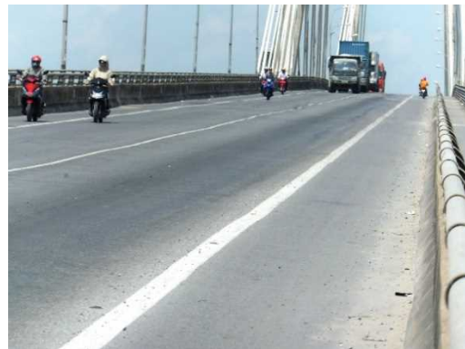
Unevenness has already appeared after repavement about 6 months earlier.
