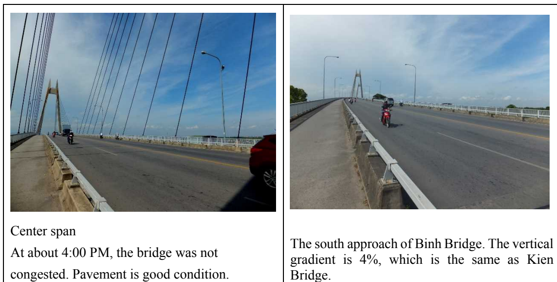
Figure 6.3-1 Pavement condition of Binh Bridge
