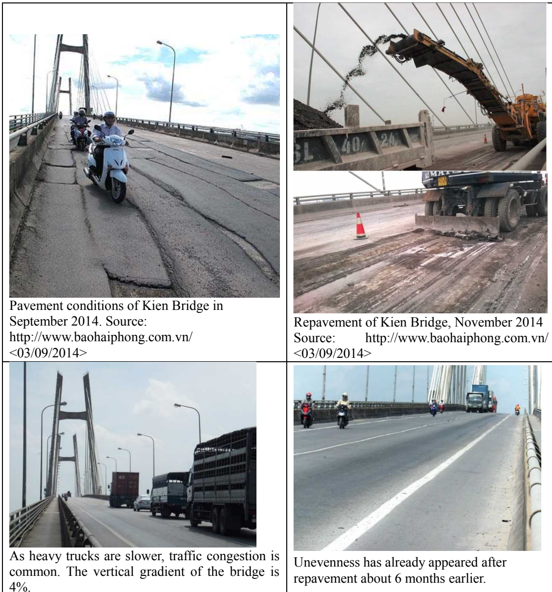
Figure 6.3-2 Pavement condition of Kien Bridge
