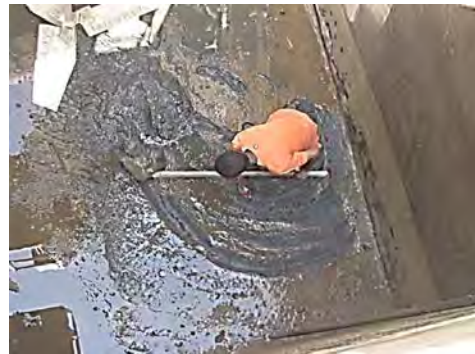
Trial of Water Quality Improvement in Toker WTP (Cleaning of Flocculation Basin)
