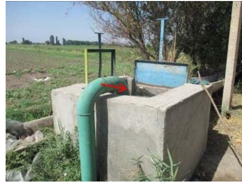
Figure A-73 Outlet of Pipe from Deep (No.39)
