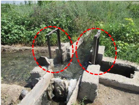
Figure A-100 Missing Gate Leaf (No.18)
