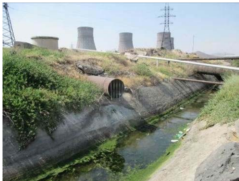
Figure A-119 Outlet of Pipe from Nuclear Power Station (No.68)
