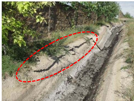
Figure A-16 Crack at Side Wall of Canal (No.26)
