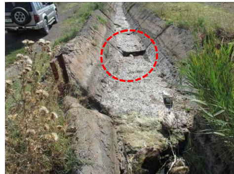
Figure A-17 Missing Portion at Bottom of Canal (No.27)
