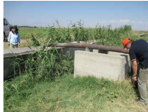
Figure A-51 Outlet of Pipe from Deep (No.29)
