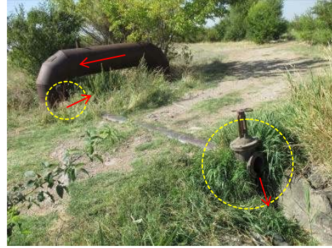
Figure A-23 Outlet ( \phi 200\text{mm} \times 2 ) of Pipe from Arzni-Shamiram Canal ( \phi 700\text{mm} ) (No.39)
