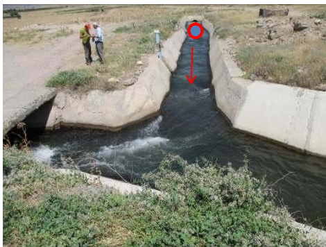
Figure A-20 Outlet of Pipe from Arizni-Shamiram Canal ( \phi 800mm) (No.25)
