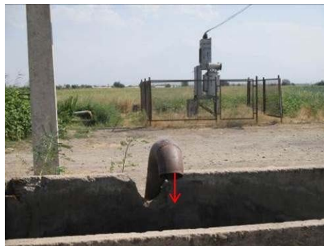
Figure A-90 Outlet of Pipe from Deep (No.30)
