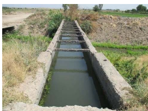
Figure A-69 Exposed Rebar at sidewall (No.23)
