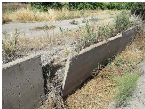
Figure A-67 Destruction of Sidewall (No.32)
