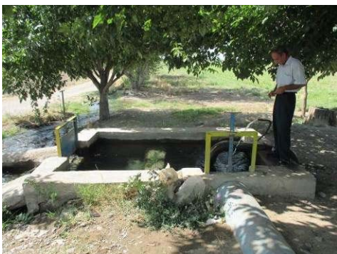
Figure A-72 Outlet of Pipe from Deep (No.36)
