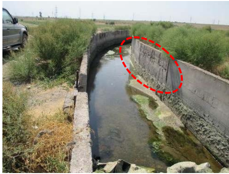
Figure A-64 Exposed Rebar at Sidewall (No.9)
