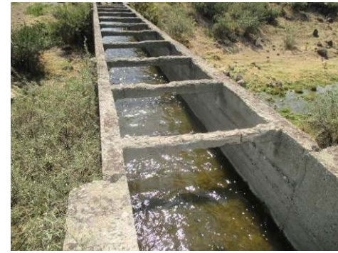
Figure A-34 Exposed Rebar at Top of Sidewall
