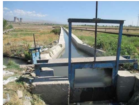
Figure A-113 Diversion from Lower Hrazdan Canal to Metsamor Canal
