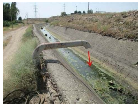
Figure A-120 Outlet of Pipe from Deep Well (No.69)
