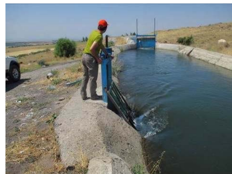
Figure A-4 Intake of pipe from Arzni-Shamiram Canal to Arzni Branch Canal
