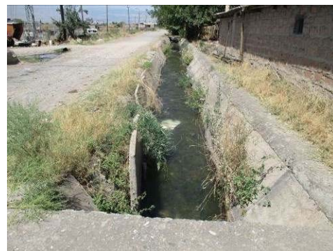
Figure A-47 Destruction of Sidewall (No.19)
