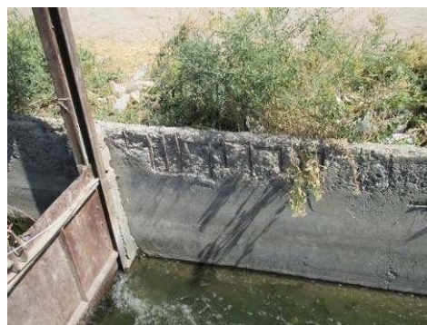
Figure A-83 Exposed Rebar at Sidewall (No.14)
