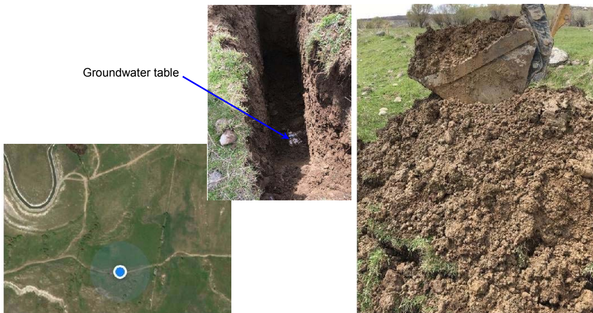
Figure 4-3-6.12 High Groundwater Table in the North Eastern Slope
