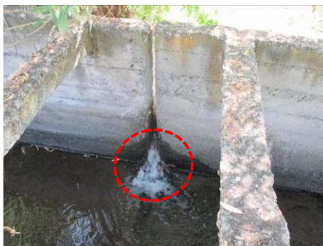
Figure 4-4-4.3 Leakage at Separation of Joint at Sidewall (No.33 )
