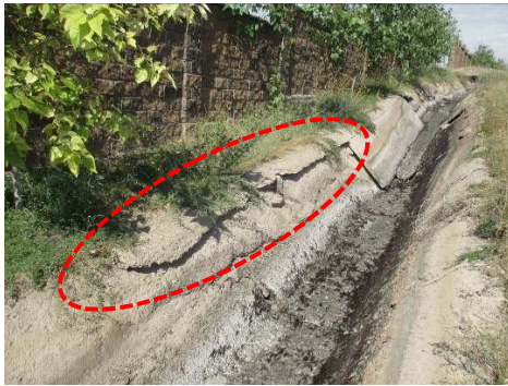
Figure 4-4-4.1 Crack at Side Wall of Canal (Arzni-Branch Canal at No.26)
