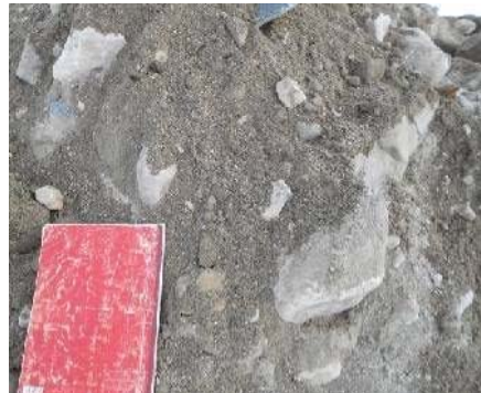
Sand-and-gravel composing the construction road lying along the foot of the north slope (TP.29)
