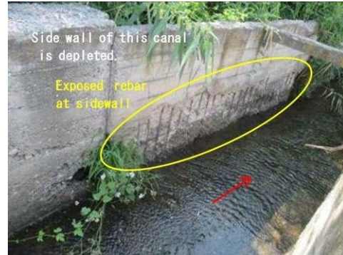
Figure A-45 Exposed Rebar at Sidewall (No.33 )
