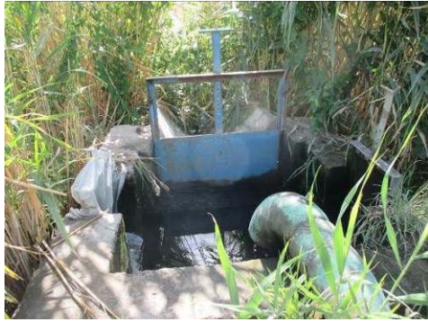
Figure A-74 Outlet of Pipe from Deep (No.40)
