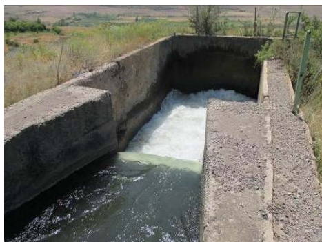
Figure A-5 Inlet of pipe from Arzni-Shamiram Canal to Arzni Branch Canal
