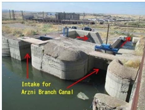
Figure A-1 Intake of Arzni-Branch Canal (No.1)
