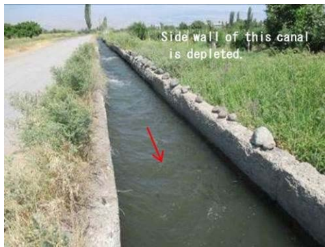
Figure A-46 Depleted Sidewall (No.9)
