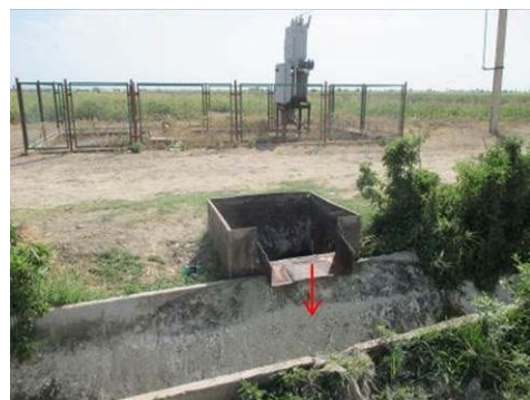
Figure A-91 Outlet of Pipe from Deep (No.34)
