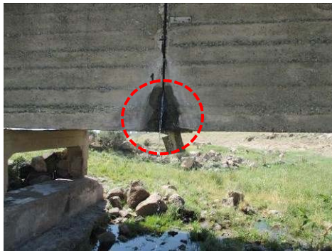
Figure A-15 Leakage from Joint at side Wall of Aqueduct Bridge (No.18)
