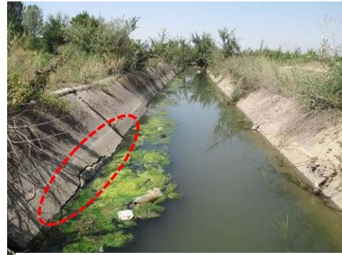
Figure A-65 Cracked Sidewall (No.22)
