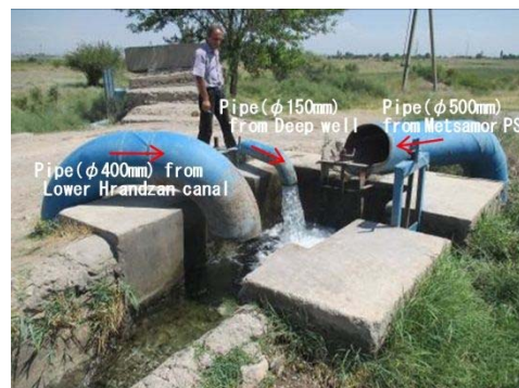
Figure A-104 Outlets of 3 Pipes from, Lower Hrazdan Canal, Deep Well Metsamo PS (No.25)
