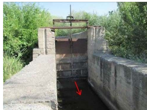
Figure A-39 Kasakh Intake (No.1)
