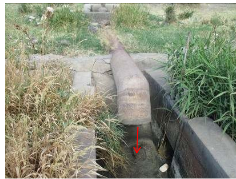
Figure A-21 Outlet of Pipe from Arzni-Shamiram Canal (φ500mm) (No.34)
