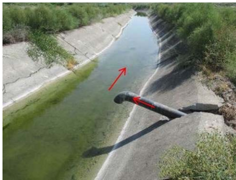
Figure A-86 Outlet of Pipe from Upper Aknalich Canal (No.5)
