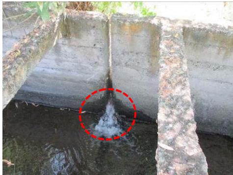
Figure A-44 Leakage from Opening of Joint at Sidewall (No.33 )
