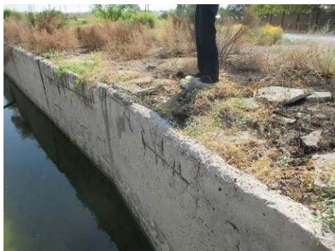
Figure A-82 Exposed Rebar at Sidewall (No.2)
