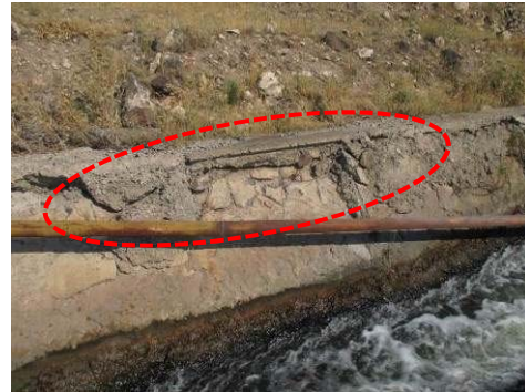
Figure A-14 Damaged Concrete at Side Wall of Canal (No.2)
