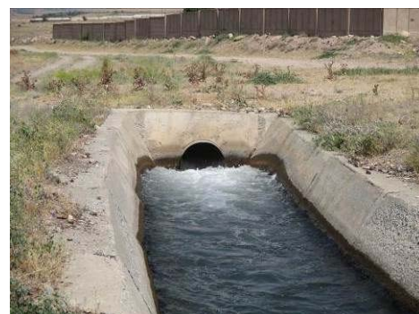
Figure A-6 Outlet of pipe from Arzni-Shamiram Canal to Arzni Branch Canal
