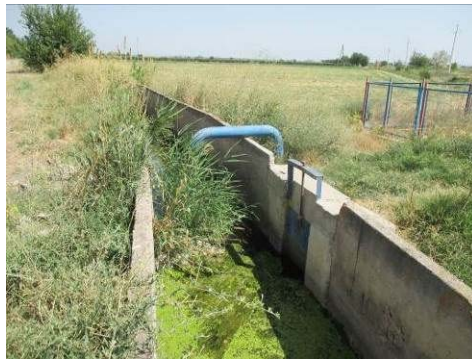
Figure A-88 Outlet of Pipe from Deep (No.24)
