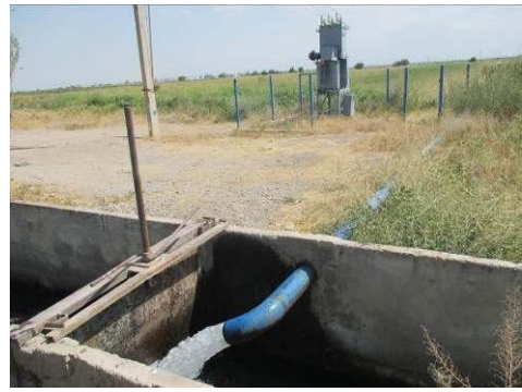
Figure A-89 Outlet of Pipe from Deep (No.28)
