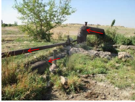
Figure A-22 Outlet ( \phi 200\text{mm} ) of Pipe from Arzni-Shamiram Canal ( \phi 700\text{mm} ) (No.37)
