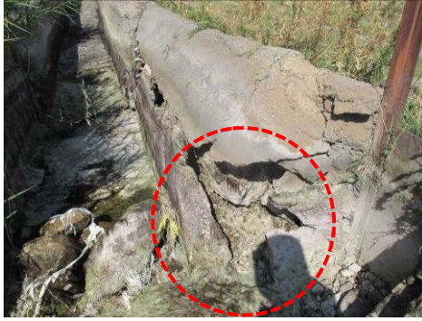
Figure A-18 Damaged Concrete at Side Wall of Canal (No.27)
