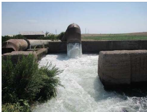
Figure A-117 Outlet of Pipe from Ranchpar No.2 PS (No.19)
