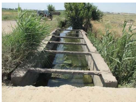
Figure A-68 Exposed Rebar at Sidewall (No.21)
