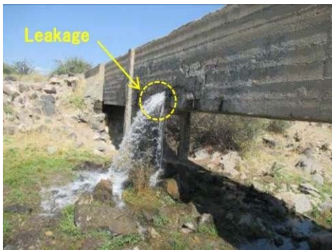
Figure A-35 Leakage from Aqueduct Bridge (No.38)
