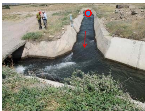
Figure 4-4-4.4 Outlet of Pipe from Arzni-Shamiram Canal (φ800mm) (Arzni-Branch Canal at No.25)
