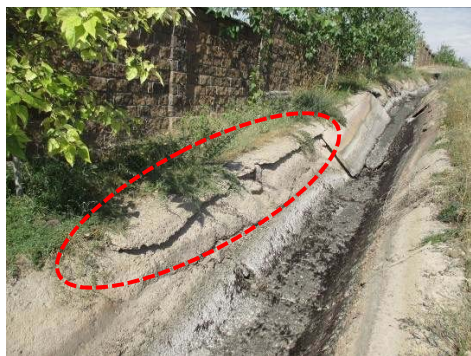
Figure 4-4-4.1 Crack at Side Wall of Canal (Arzni-Branch Canal at No.26)
