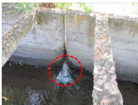
Figure 4-4-4.3 Leakage at Separation of Joint at Sidewall (No.33 )
