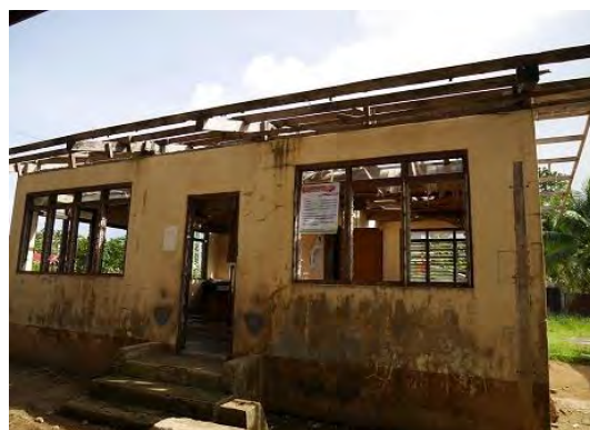
Figure 5- 12 BHS destroyed by Typhoon Ruby
