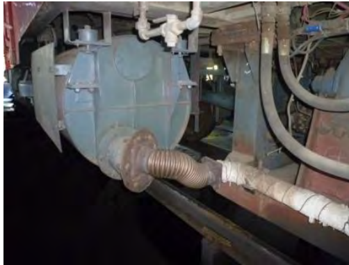
Kinked exhaust pipe
