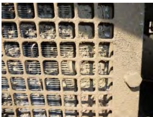
Clogged filter (cause of overheating)
