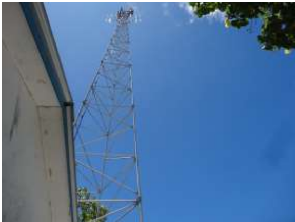
Existing antenna tower at the site in Ungoofaaru
