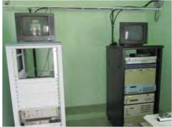
Equipment for analogue broadcasting and FM radio at the station in Villingili
