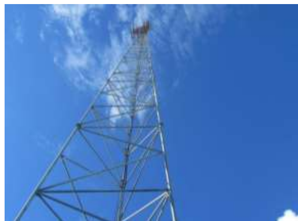
Existing antenna tower for analogue broadcasting at the site in Thinadhoo
