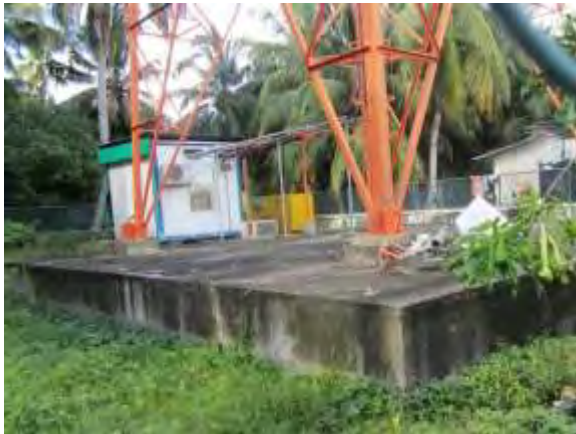
Existing foundation for analogue broadcasting tower and station building at the site in Fiyori
