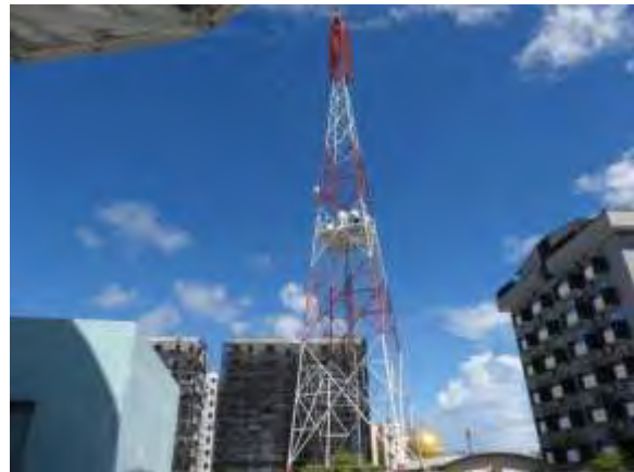
Existing antenna tower for analogue broadcasting at PSM
