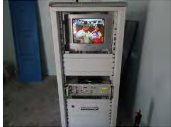
Equipment for analogue broadcasting at the station in Manadhoo
