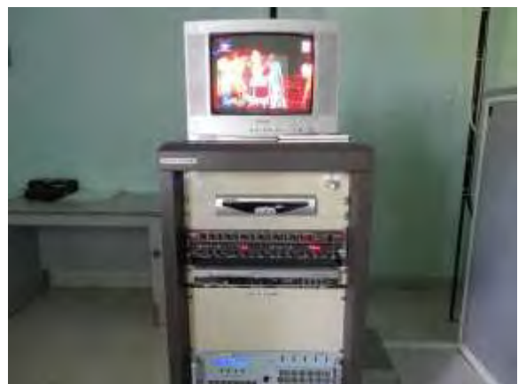
Equipment for analogue broadcasting at the station in Eydhafushi
