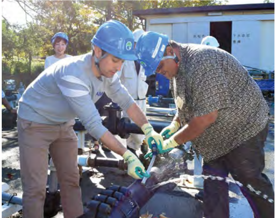
Training participants learning a repair technique for water leakage at a training facility in Hamamatsu City, Shizuoka Prefecture: Knowledge Co-Creation Program (Group and Region Focus) — Non-revenue Water Management (Leakage Control)
