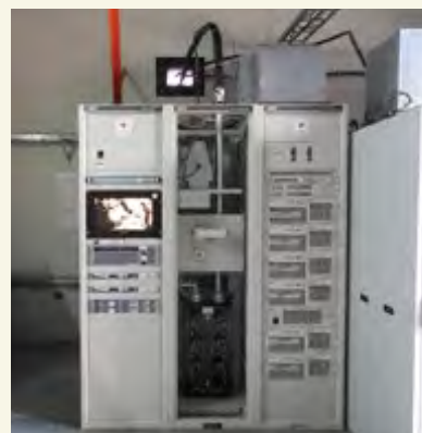
EWBS digital transmission equipment (Photo: Yachiyo Engineering Co., Ltd.)
