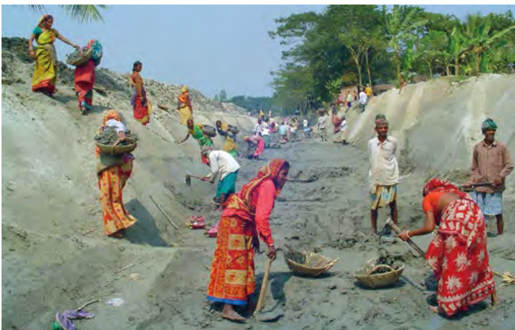
An ODA Loan project in Bangladesh provides the opportunity for local poor people to be employed and earn money doing daily rural road maintenance. The project saves part of their wages in bank accounts that they can use to buy livestock, start small stores, etc. when their employment is over.
