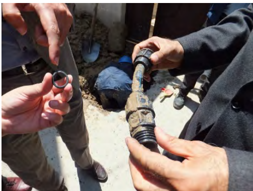
Leak Repair (Degraded Rubber Ring)
