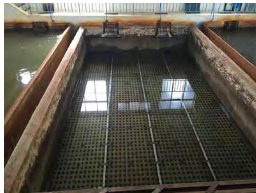
Jalailah Water Treatment Plant
