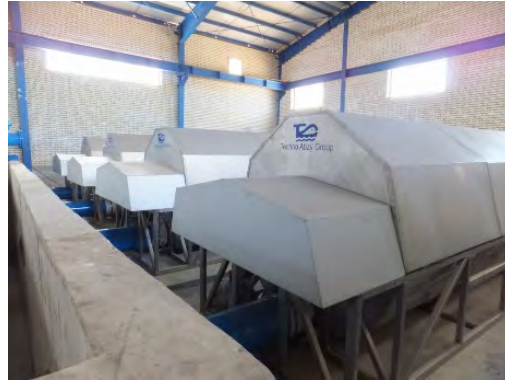
Water Treatment Plant (Strainer Equipment)
