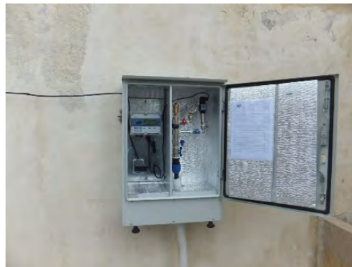
Water Pressure Monitoring Equipment (At Mosque)
