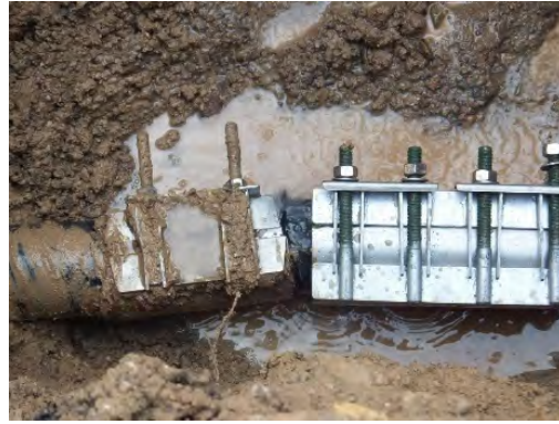
Leak of Distribution Main (Crack in PE Pipe)
