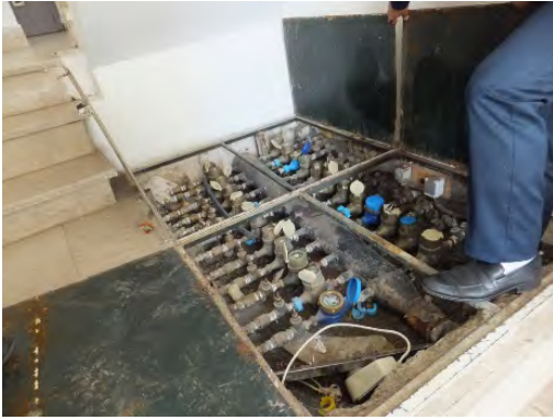
Housing Complex Water Meters (Individual Type)
