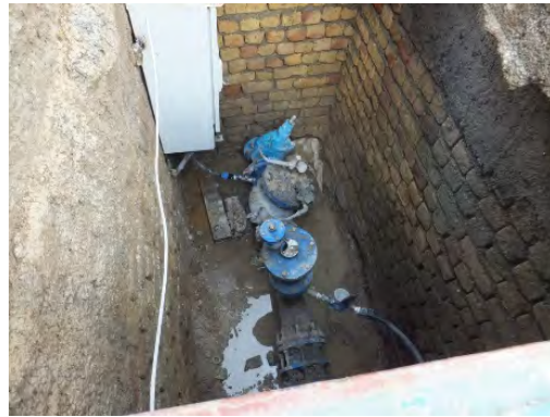
PRV (Inside the Valve Chamber)
