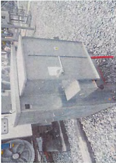
Neutral Grounding Resistor
