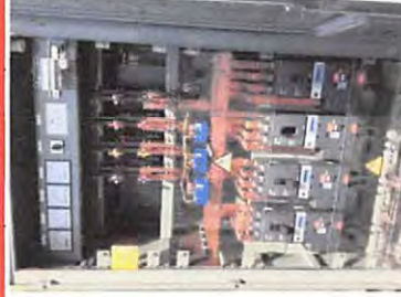
MCCB (installed in the distribution box)
