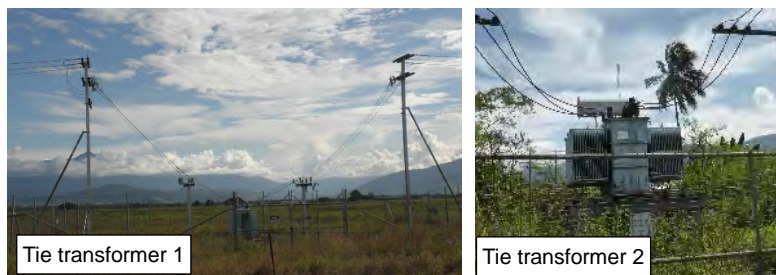
Fig. 2.3-14 Photographs of the Tie Transformers
