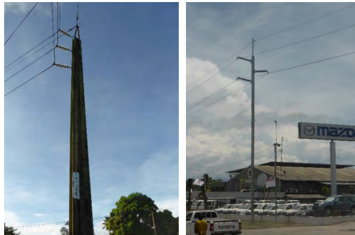
Fig. 2.1-3 Photographs of 66kV Transmission Lines
