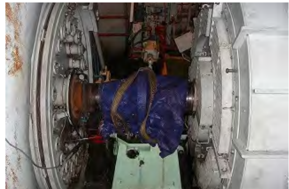
Unit #2 Turbine: damaged turbine bearing
