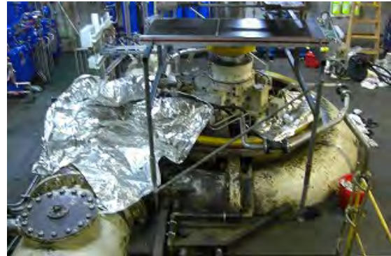
Unit #3 turbine: out of order
