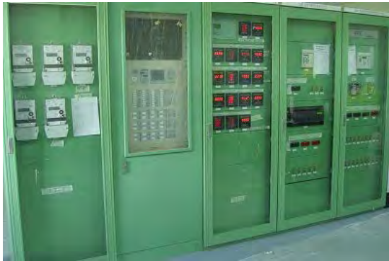
Control Room In
