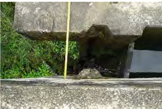
Gap of forebay structure
