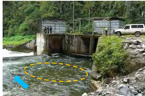
Intake: Abundant sediment materials are deposited in front of the Intake.
