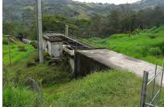
The forebay is unstable due to sliding and settlement.
