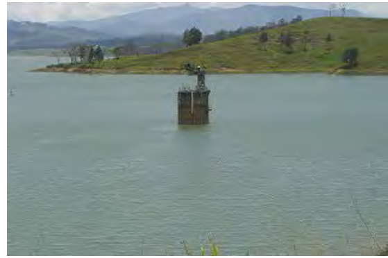
YTOD Hydropower: Intake tower gate
