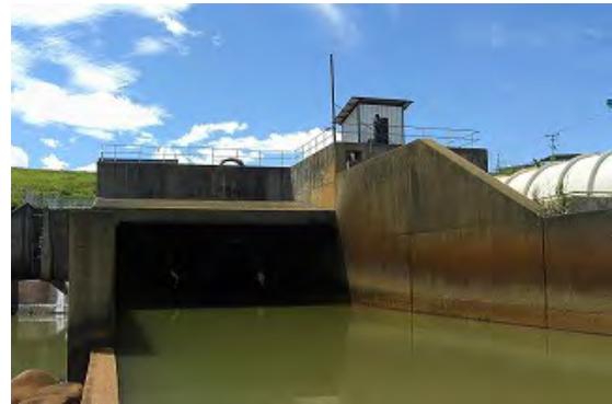
Outlet of Bypass valve
