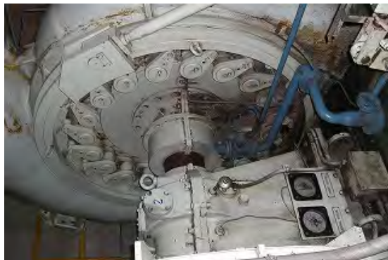
Unit #1 Turbine: failure of water cooling system
