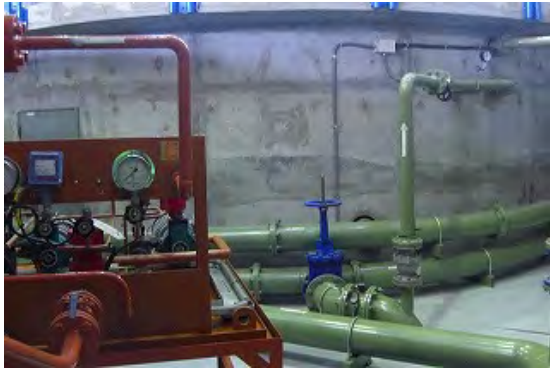
Water supply system: it functions insufficiently
