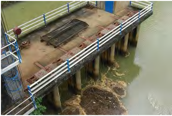
Intake: The intake screen is blocked by a lot of debris.
