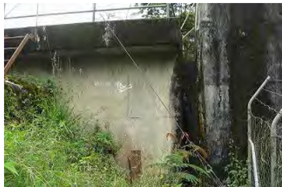
Gap of forebay structure
