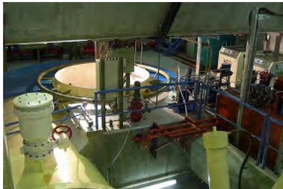
Turbine and generator
