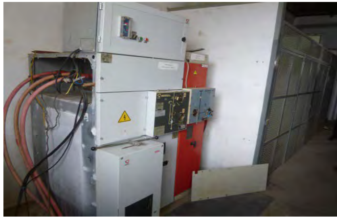
20kV switchgear (left: by EFACEC, center: by ALSTOM) and transformer (back right)
