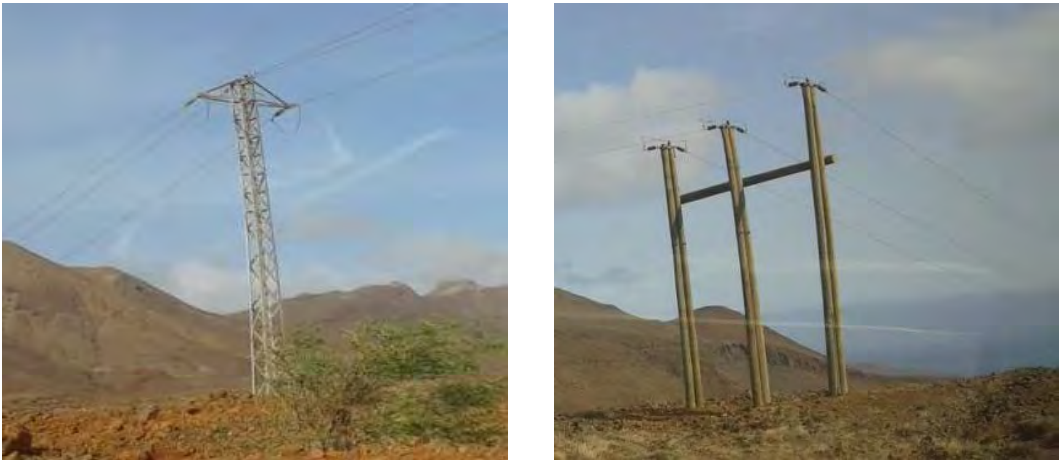
Figure 9.1-7 20kV Transmission facilities (between R.Brava and Cacimba PS)
