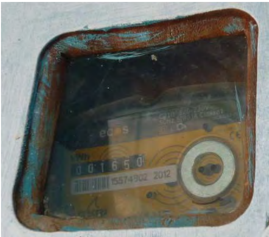
Figure 9.1-25 Residential electric power meter
