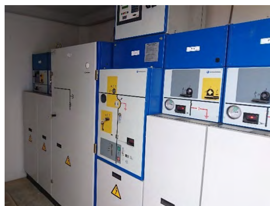
(b) Power source connection panel (PS)
