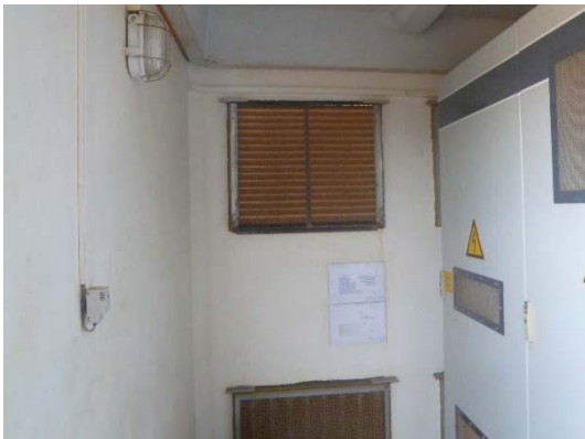
(e) PT external air suction inlet
