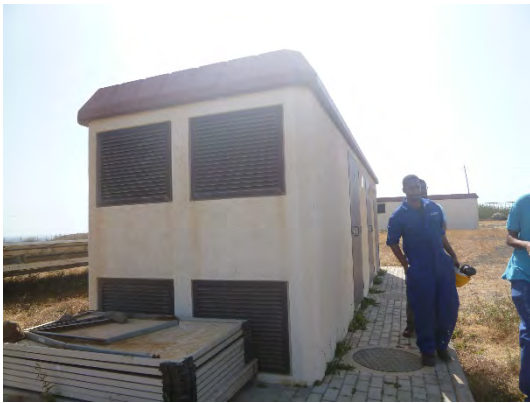
(c) Inverter, transformer hut (PT)
