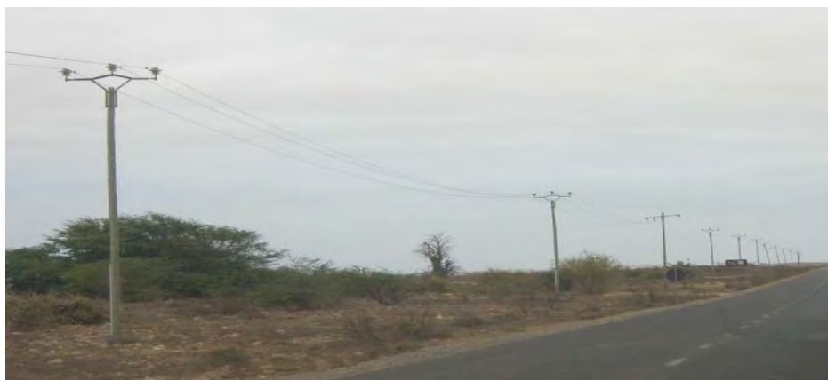
Figure 9.1-15 20kV overhead transmission line in the north-western region
