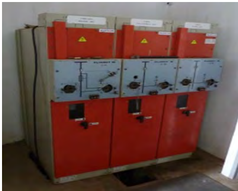
6kV switchgear (by ALSTOM) (two feeders)
