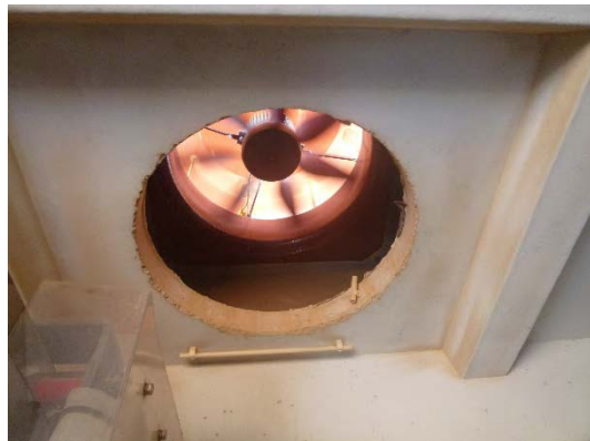
(f) PT exhaust vent
