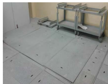
Space for extra 20kV switchgears
