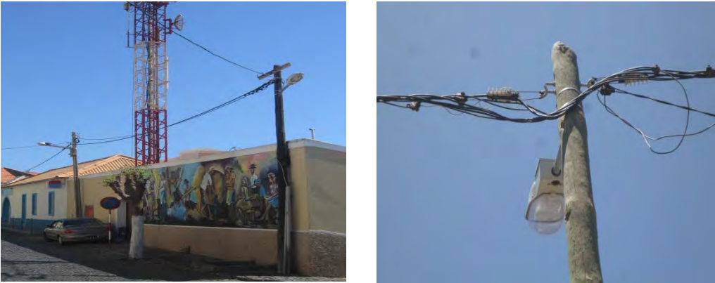
Figure 9.1-24 Low Voltage distribution lines
