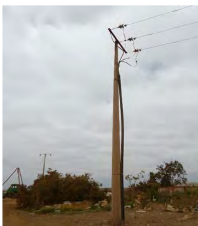
Figure 9.1-13 10kV line leading-in pole at F.d.figueiras
