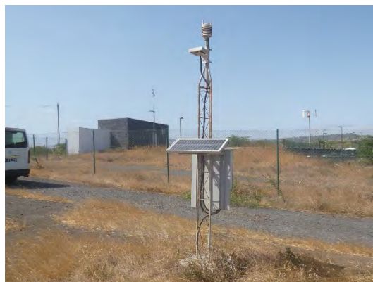
Figure 8.1-8 Weather Data Observation Equipment (Santiago)
