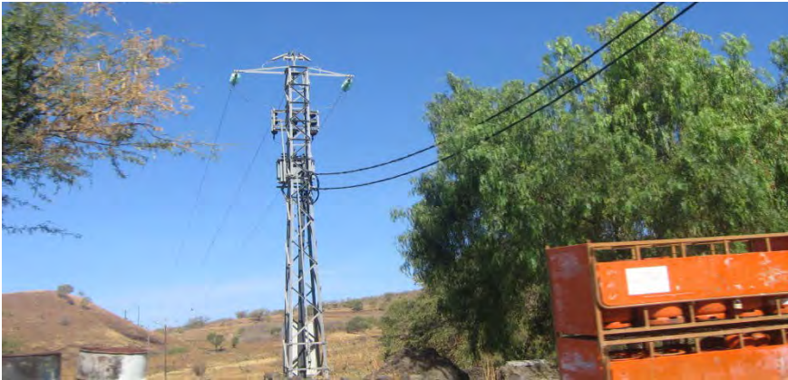
Figure 9.1-23 Steel tower with a transformer
