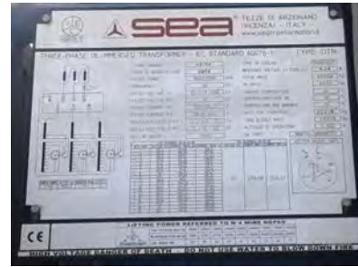
Transformer nameplate (made in Italy)
