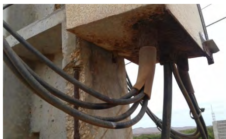
Close-up of the cable box (severe corrosion due to rust)
