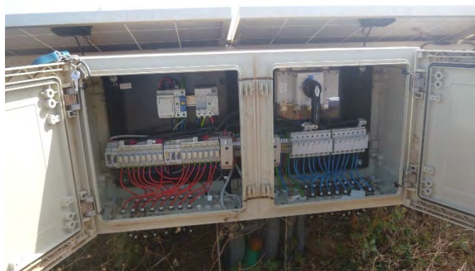
Figure 8.1-18 Junction Box (Santiago)
