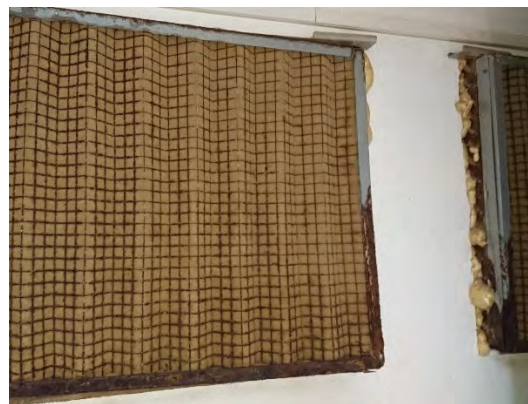
(b) Building ventilation fan filter
