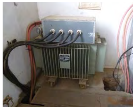
House transformer: 250kVA (by GONELLA) (20kV/400V)
