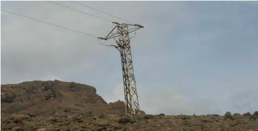
Figure 9.1-8 20kV underground cable leading-in steel tower (between C.Norte and Juncalinho)
