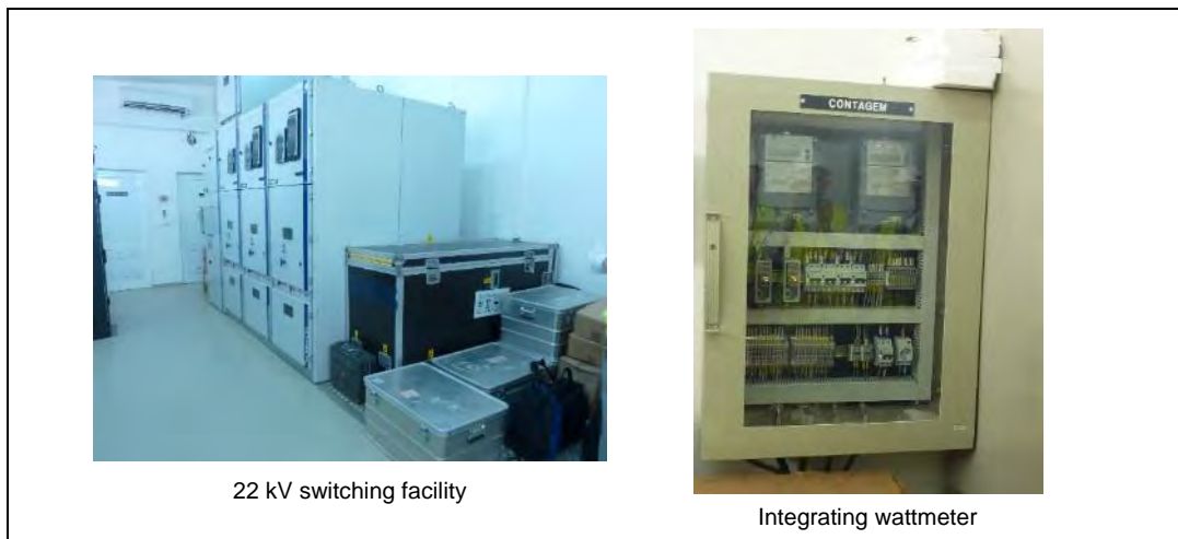
Figure 7.1-13 Conditions of the grid connection facilities
