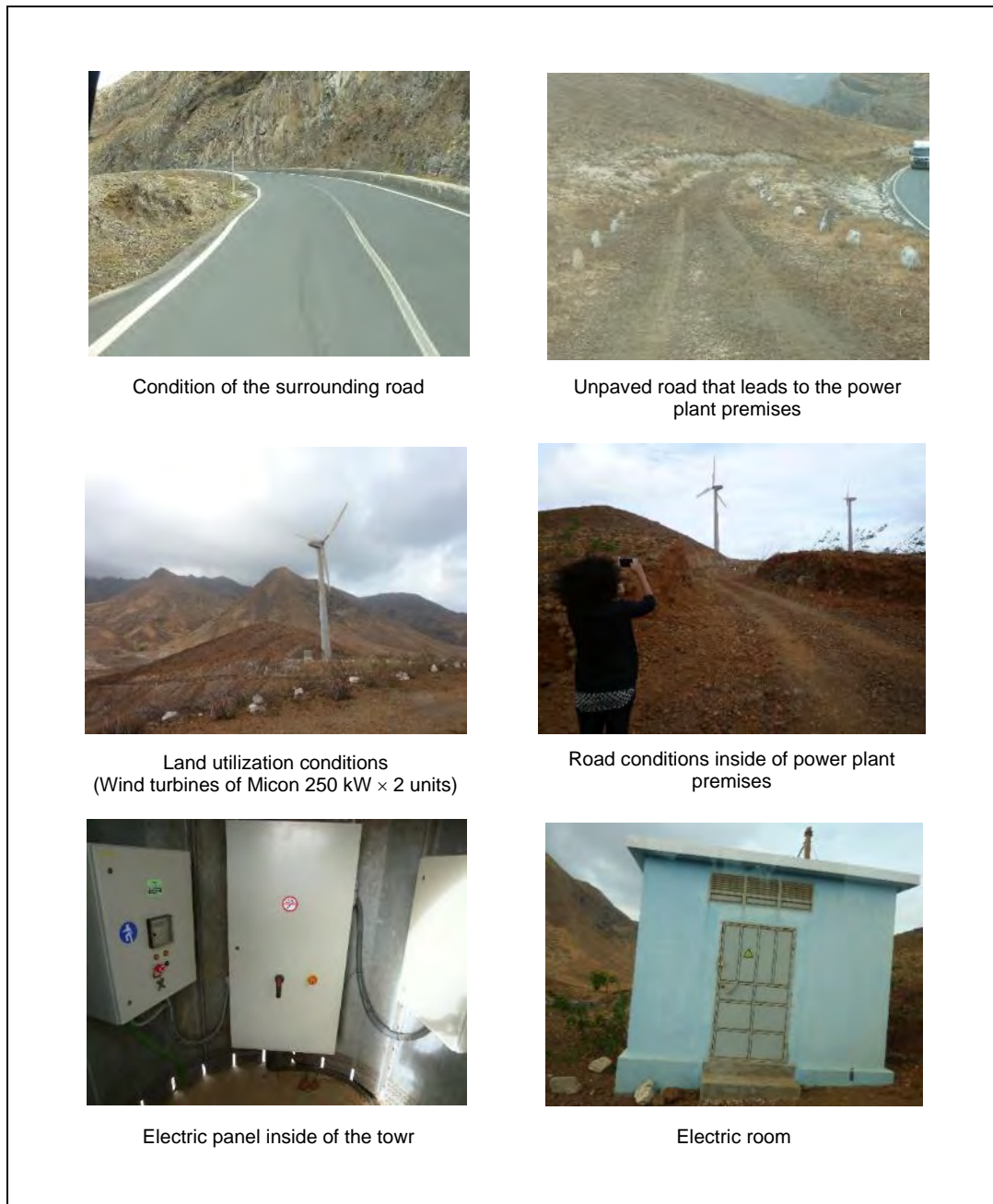
Figure 7.1-32 Conditions of the Santo Antão wind power generation system
