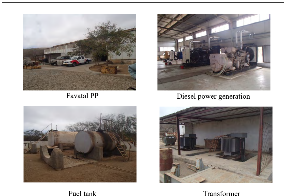
Figure 6.1-9 Diesel power facilities of Brava
