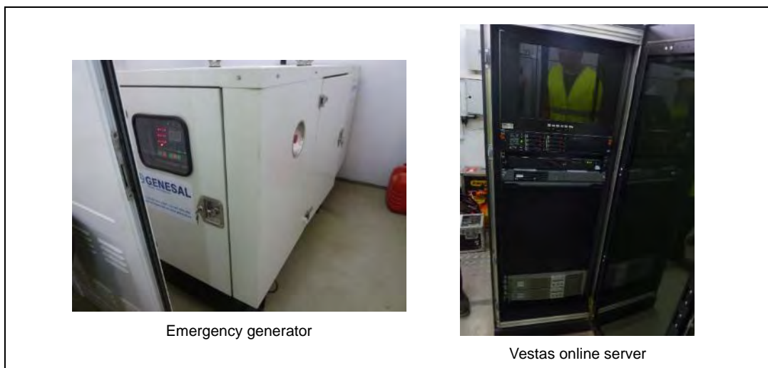
Figure 7.1-14 Conditions of the electrical facilities
