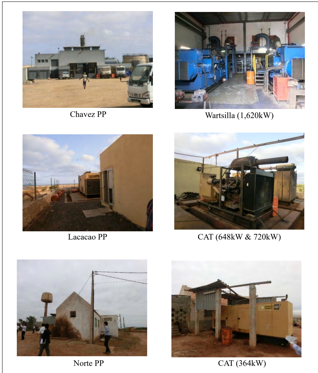
Figure 6.1-5 Diesel power facilities of Boa Vista
