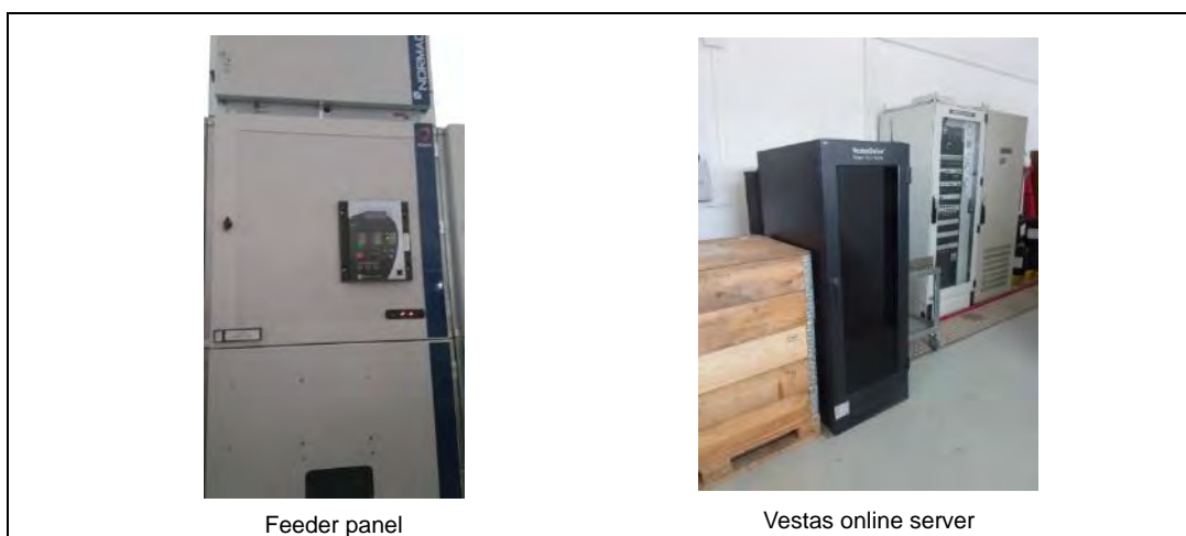
Figure 7.1-12 Conditions of the electrical facilities
