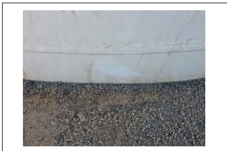
Figure 7.2-1 Condition of the repairs at the bottom of the tower (Boa Vista)
