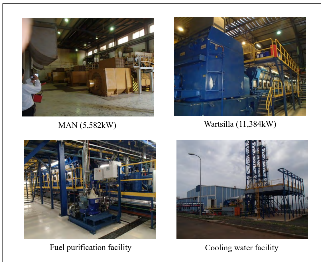
Figure 6.1-7 Diesel power facilities of Santiago
