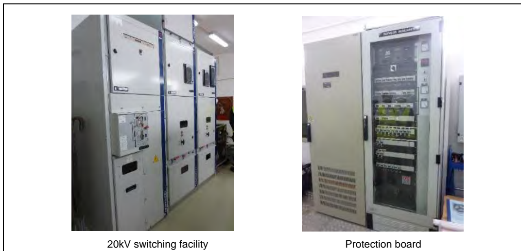
Figure 7.1-15 Conditions of grid connection facilities
