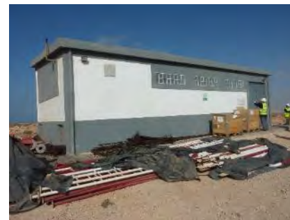
Control building (Electric room)
