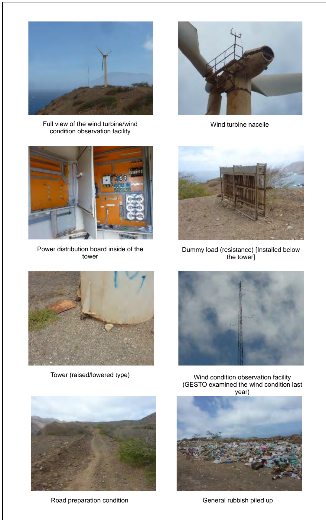
Figure 7.1-35 Condition surrounding the Brava wind power generation system
