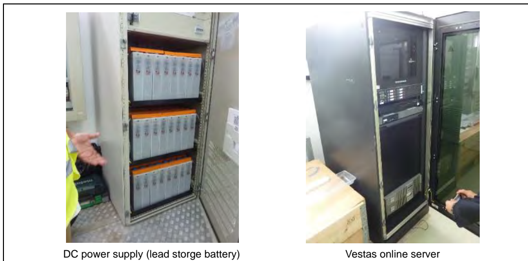
Figure 7.1-16 Conditions of the electrical facilities
