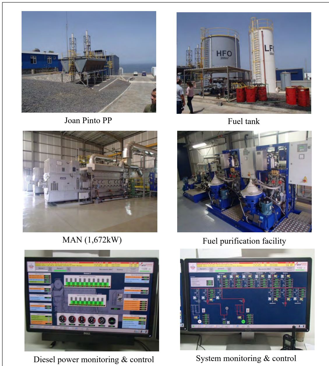
Figure 6.1-8 Diesel power facilities of Fogo
