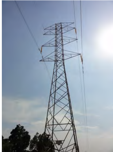
Photo 3-2-4.1 Transmission line between Nalubaale Substation, Namanve Substation and Kampala North Substation
