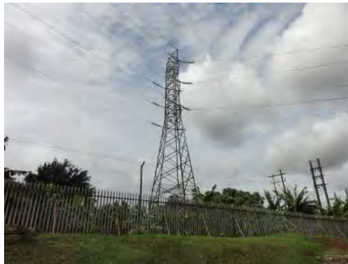
Photo3-2-4.4 Transmission line between Kampala North Substation and Lugogo Substation
