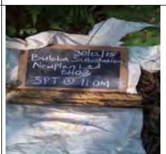
SPT at 11m for BH3, moist mottled brownish yellow firm intact silt of high plasticity, elastic silt
