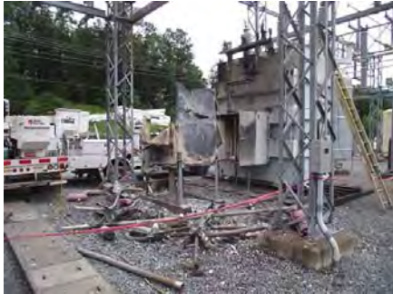
Figure 7-12: Example of damage caused by a snake at a substation Source: http://tdworld.com/substations/protect-your-substations-against-animal-intruders
