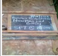
SPT at 15m for BH4, moist mottled greyish yellow stiff intact silt of high plasticity, elastic silt
