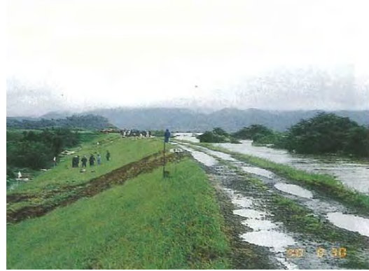
b) Water Pools on Dyke Crown
