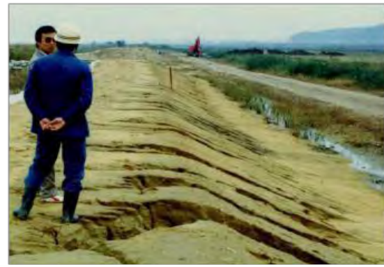
d) Erosion (Gully) due to Rainfall
