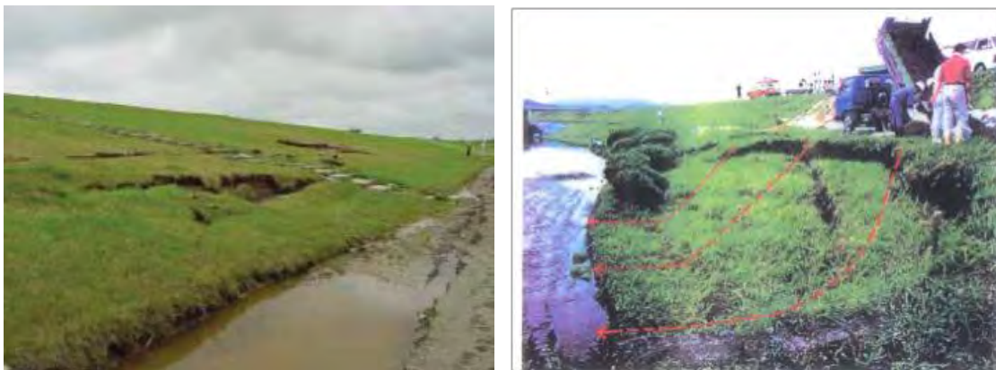
d), e) Slope Failure and Fluidization
