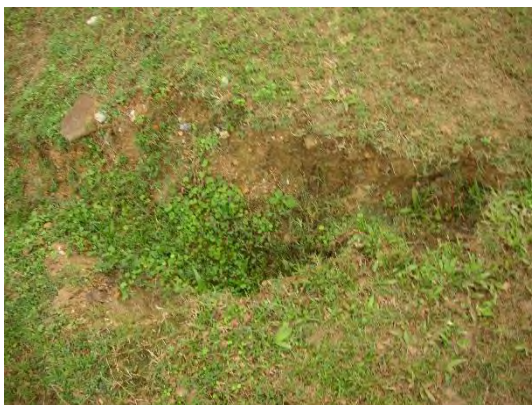
f) Caving of Slope
