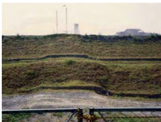
i) Slip up around Crossing Structures
