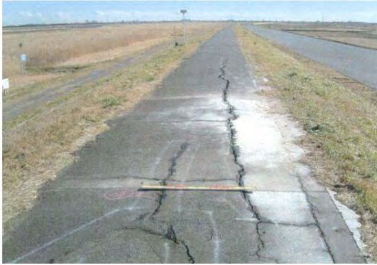
a) Crack on the Dyke Crown
