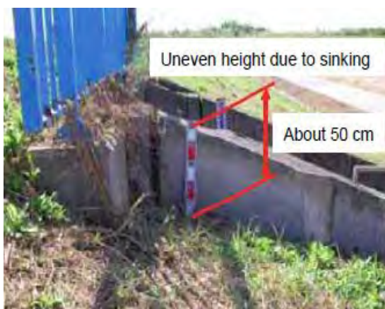
h) Uneven Height by Sinking
